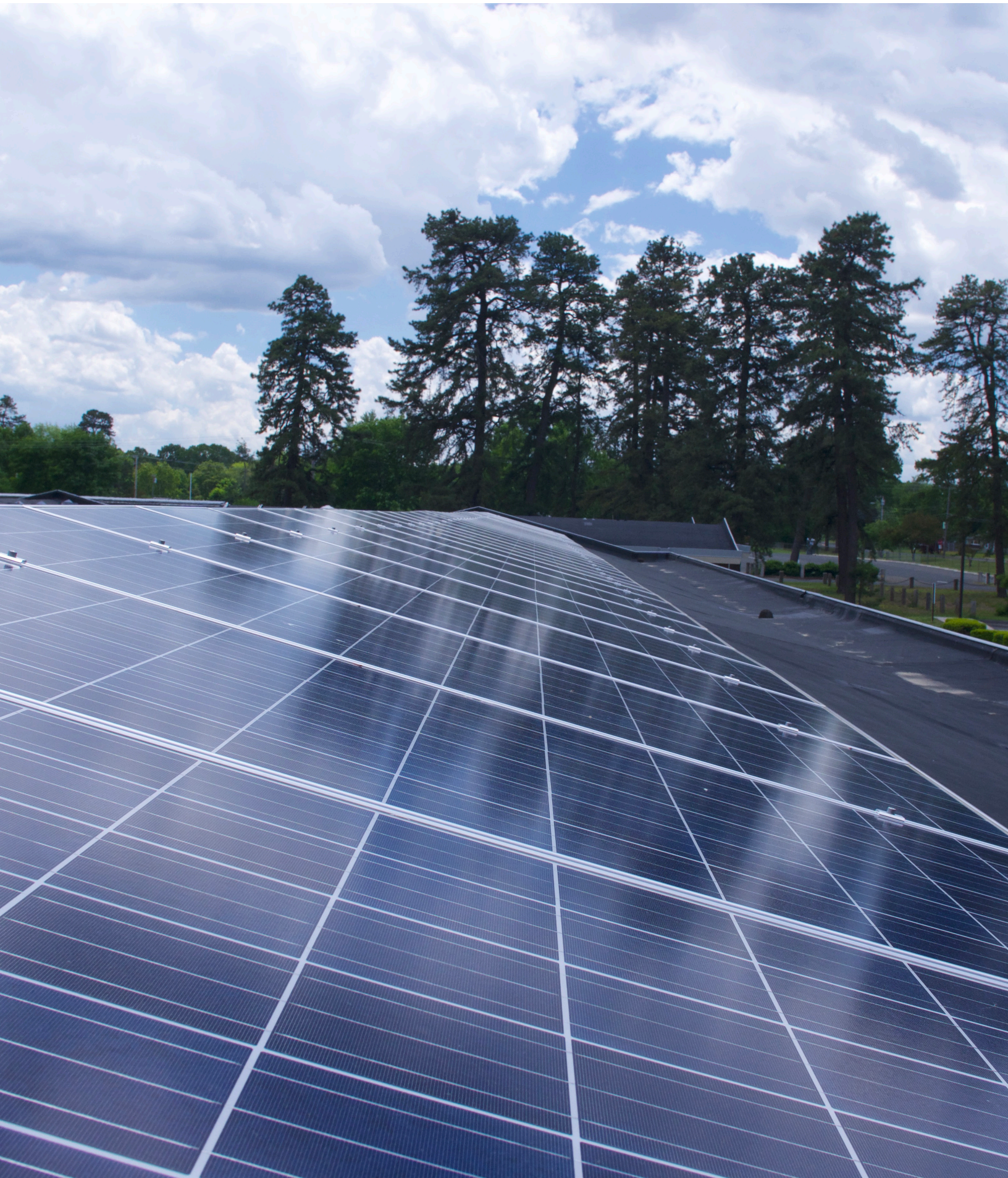
Solar panels on the roof of an affordable multifamily property in Windsor Locks.
